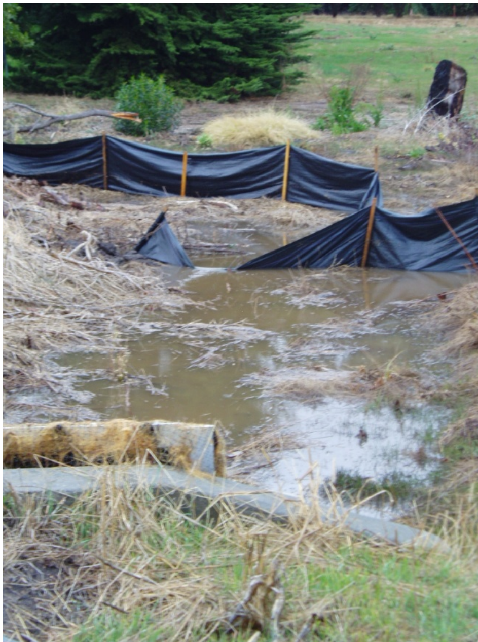
Channelkeeper documented failing erosion and sediment control measures in a storm in 2007.
